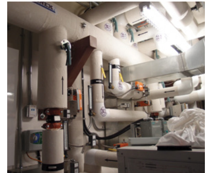
Figure 4. HVAC pipe insulation
