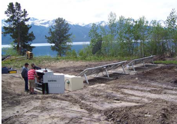
Figure 7. The Xenig Gwet'in PV/genset/battery hybrid
