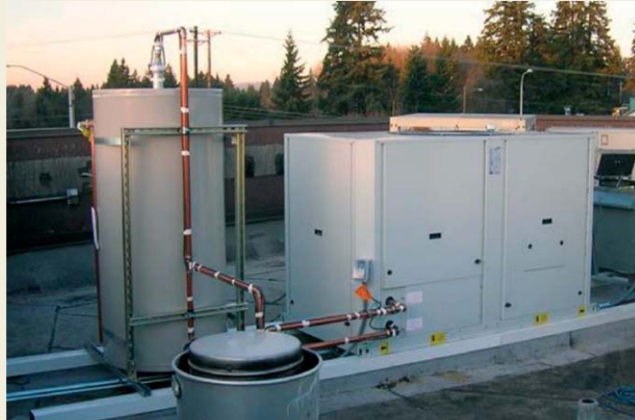
Figure 3 – Carrier 60kW CO 2 Heat Pump installed on restaurant roof in Oregon
