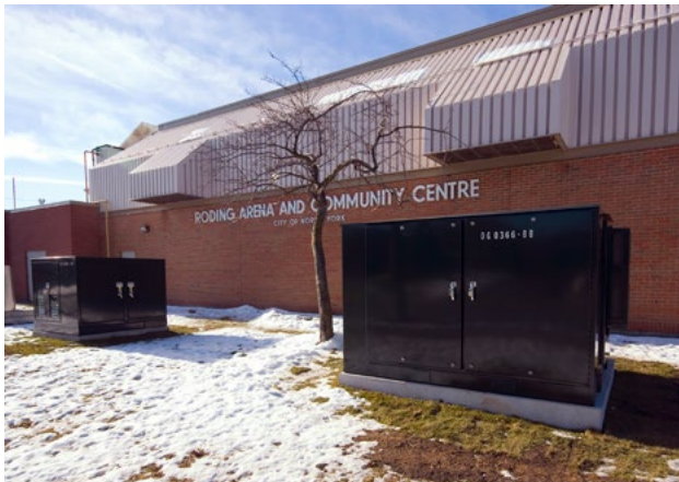
eCAMION's 500 kW/ 250 kWh community energy storage project with Toronto Hydro
