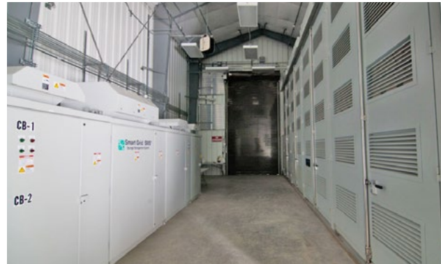
BC Hydro Field substation battery controls
