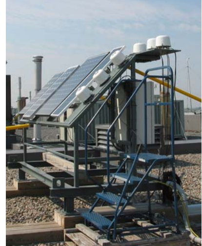
PV module outdoor test platform CanmetENERGY research facility, Varennes
