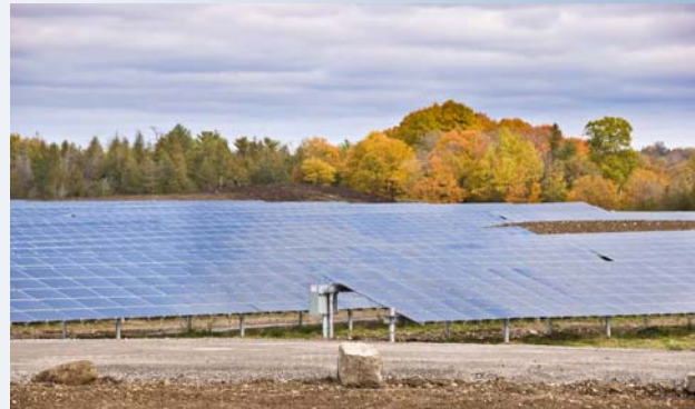
Figure 1 : SunEdison's and SkyPower Corporation's 9.1-megawatt (MW) First Light Solar Energy Park in Stone Mills, Ontario, and the largest solar energy park built to date in Canada. (Photo credit: Dave Turcotte, CanmetENERGY)
