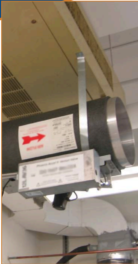
Laboratory room supply air valve
