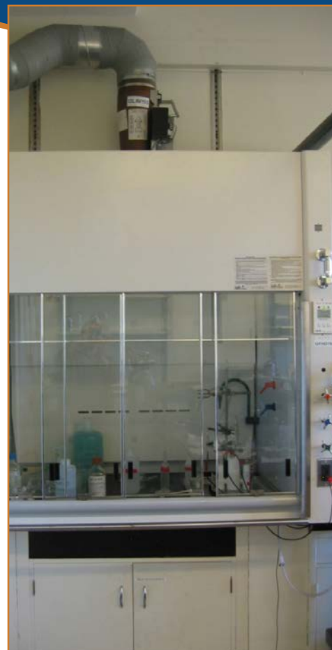
New high efficiency/low airflow fume hood
